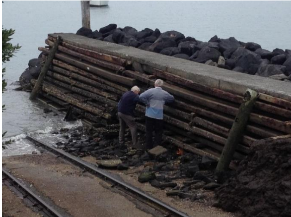
John and Chris discuss the state of the sea wall
